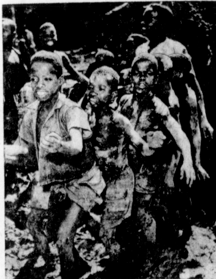
DIRTY WORK AFOOT —Mothers and teachers normally frown on kids who play in mud, but these Liberian schoolboys have full approval for their dirty work. In rhythm to a song they're singing, the boys are tromping out mud to make mud blocks for the construction of a new village school at Dingama.
