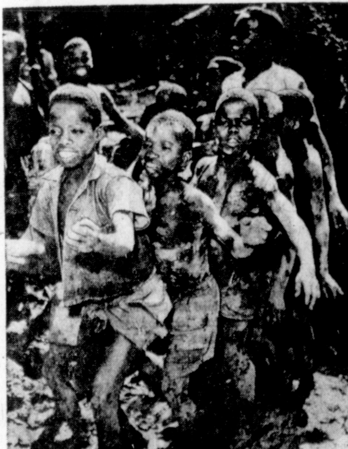
DIRTY WORK AFOOT —Mothers and teachers normally frown on kids who play in mud, but these Liberian schoolboys have full approval for their dirty work. In rhythm to a song they're singing, the boys are tramping out mud to make mud blocks for the construction of a new village school at Dingama.
