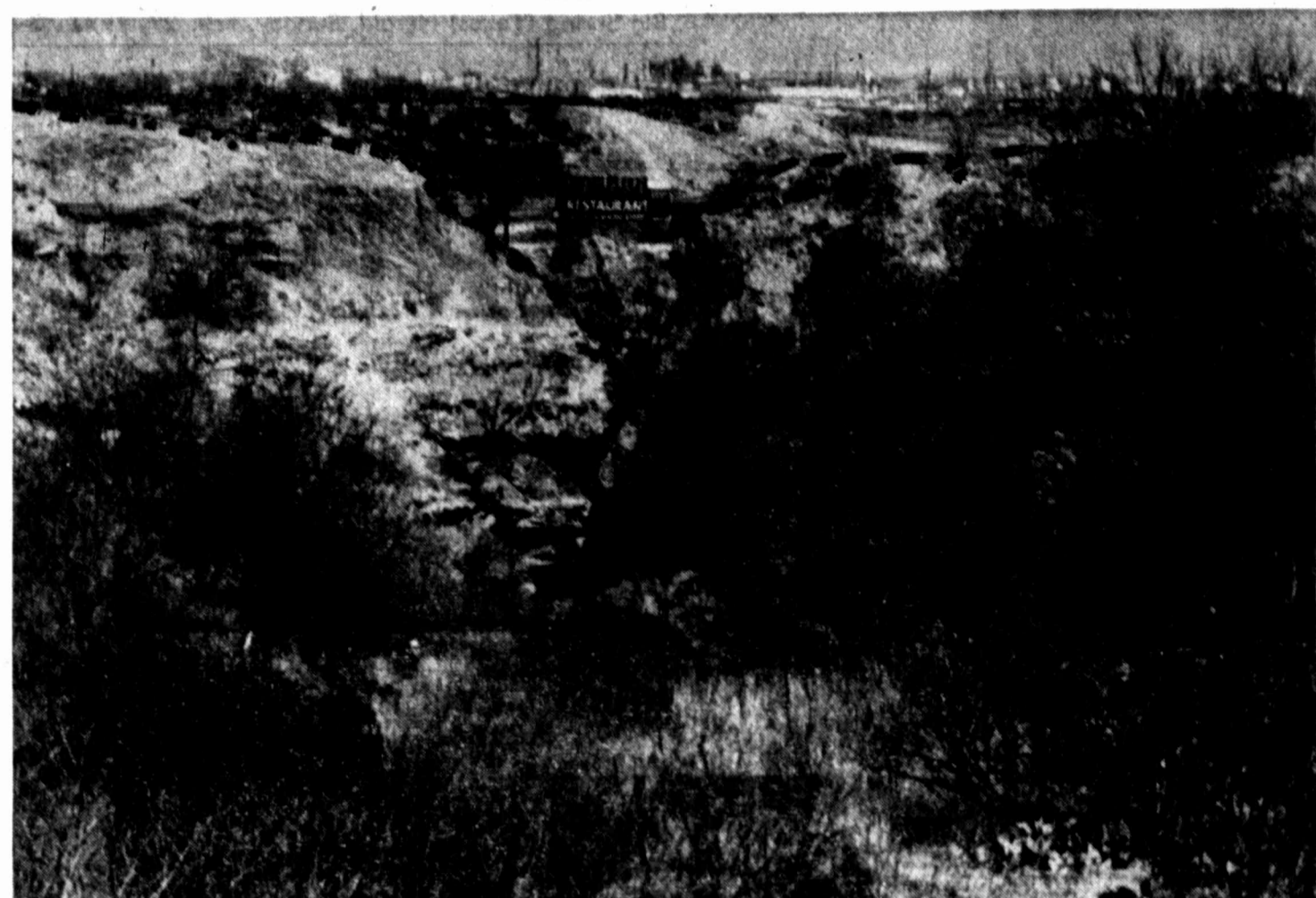
VIEW OF BROKEN DAM LOOKING EASTWARD ACROSS GOLIAD STREET Dotted lines mark outline of break in old dike
