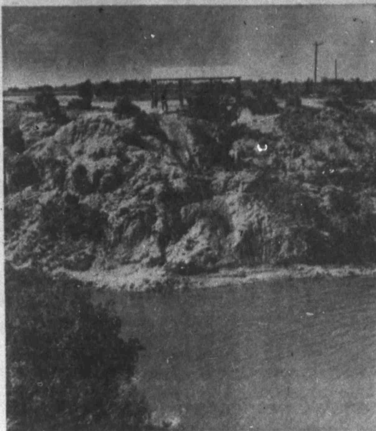
EASIER ACCESS TO WATER'S EDGE Workmen getting ready to build concrete steps
