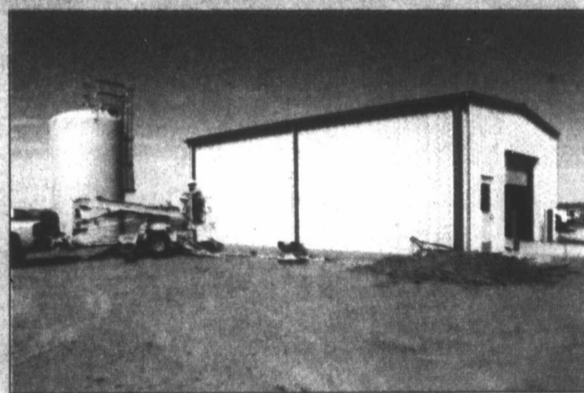
MAKING FRESH WATER - The desalination plant in the western part of the county is under construction and will produce 250,000 gallons of fresh water from brackish water everyday once in operation.
