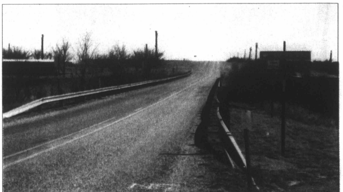
BRIDGE REPLACEMENT - The bridge spanning Cherry Creek on FM 2836 is going to be replaced by the Texas Department of Transportation in the very near future. Travelers crossing the bridge may have to deal with detours while the bridge undergoes construction.
