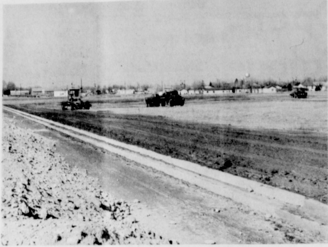
WORK PROGRESSES — Shown above is some of the work just completed and some just started in the Highland Addition of Floydada. The curbing had been completed and the gravel had been piled in the road in preparation for paving. The property is owned by John Key West. (Staff Photo)
