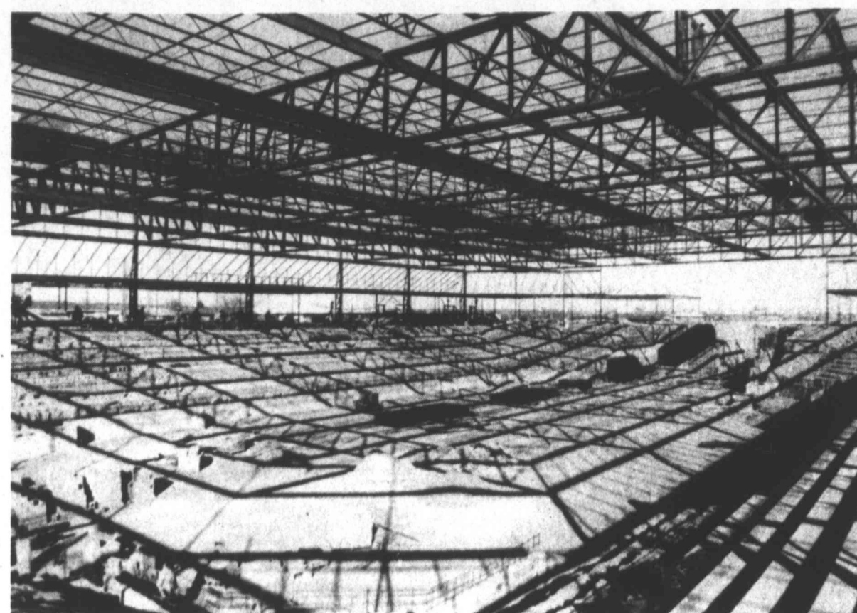
SHADOWS OF PROGRESS — Shadows from the rafters in the coliseum going up at Howard College reflect across the main area of the building as construction continues at the facility. The sunny winter days, which account for the shadows of the rafters, also add to working days which may make the completion of the facility come early in the fall.
