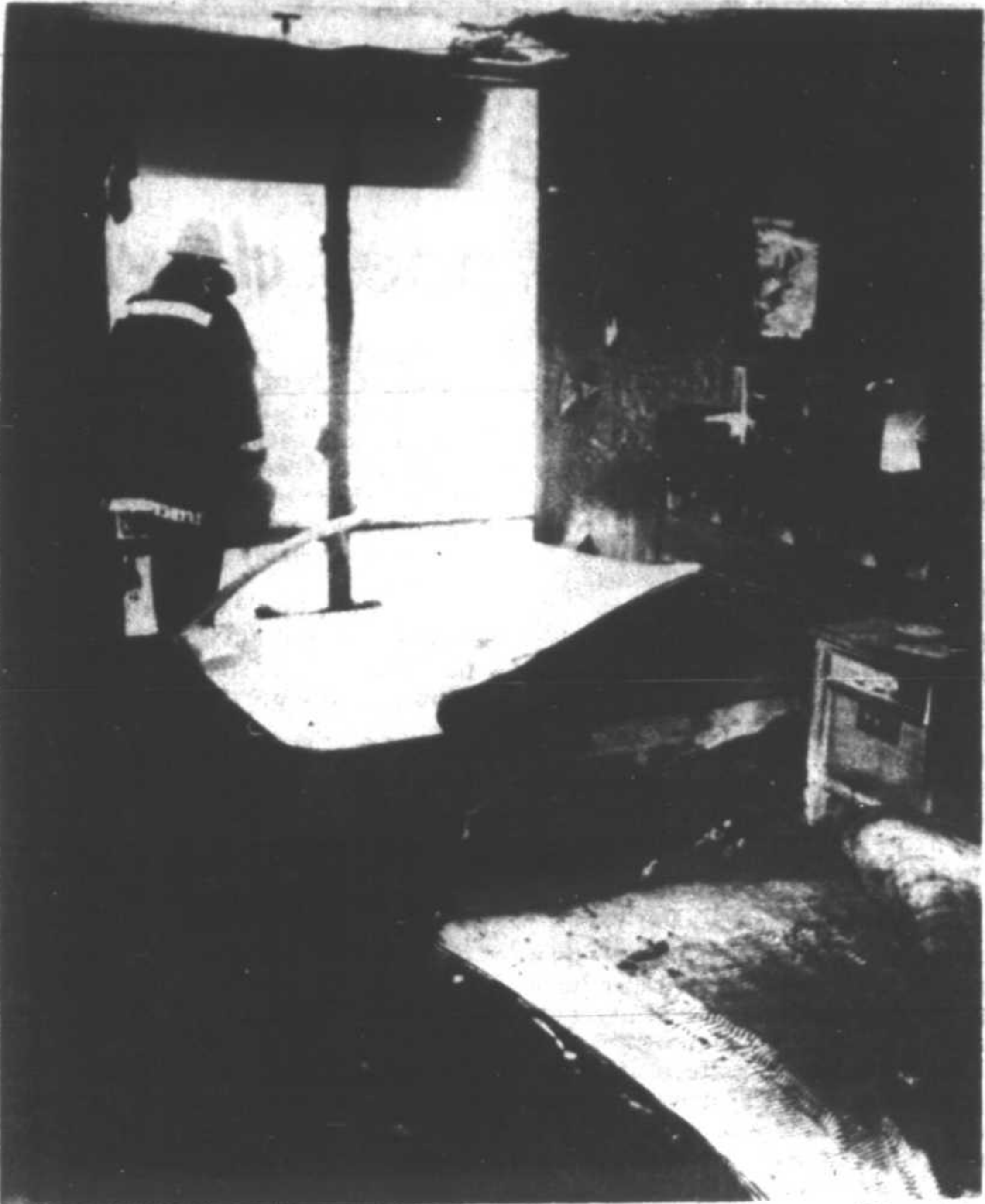
Fire inspector Joe Walker looks out the window of one of the heavily damaged rooms after a two-alarm fire hit the Hilton Hotel in Tulsa, Okla., Sunday afternoon. Two guests, Mr. and Mrs. Steve Avery of Corpus Christi, were treated and released from a local hospital for smoke inhalation.
