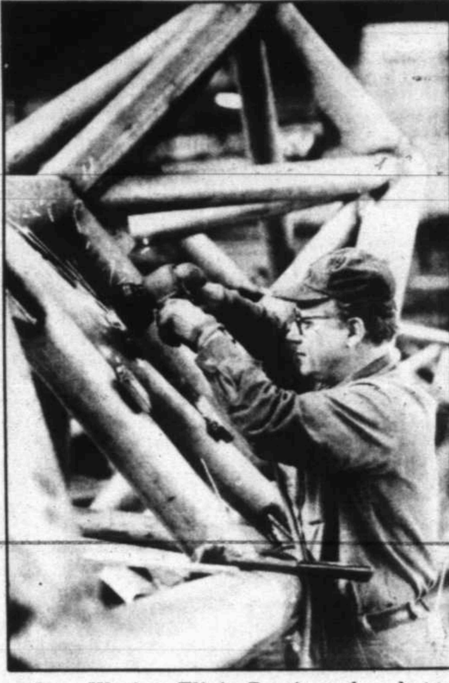
Iron Worker Eligio Perti sands a brace on the Isamu Noguchi sculpture honoring Benjamin Franklin. Perti and his co-worker Joseph DiNardi are constructing the sculpture, consisting of a kite, a key, and a lightning bolt, and is expected to be placed this spring on the Philadelphia side of the Ben Franklin Bridge spanning the Delaware Bridge.
