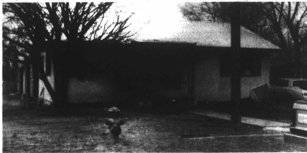
FIRE DAMAGED: Units of the Colorado City Volunteer Fire Department responded in the early morning hours to the Garcia residence at 403 Cypress in the early morning hours of Tuesday, Dec. 17. The cause of the fire that began in the bedroom remains under investigation.
