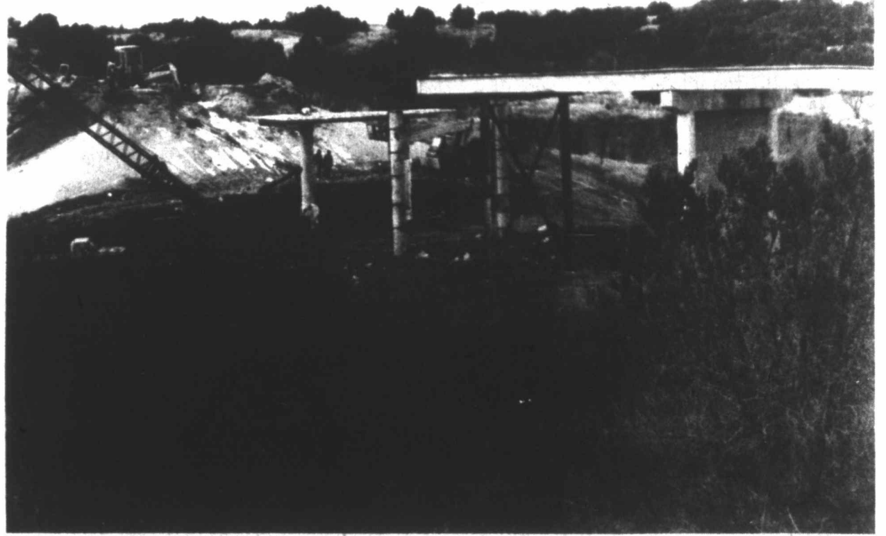
BRIDGE WORK - Construction is underway on a new bridge to span the Colorado River on Farm to Market Road 1808 in northern Mitchell County. A temporary crossing has been built while construction on the new bridge, which will be wider than the older one, is underway.
