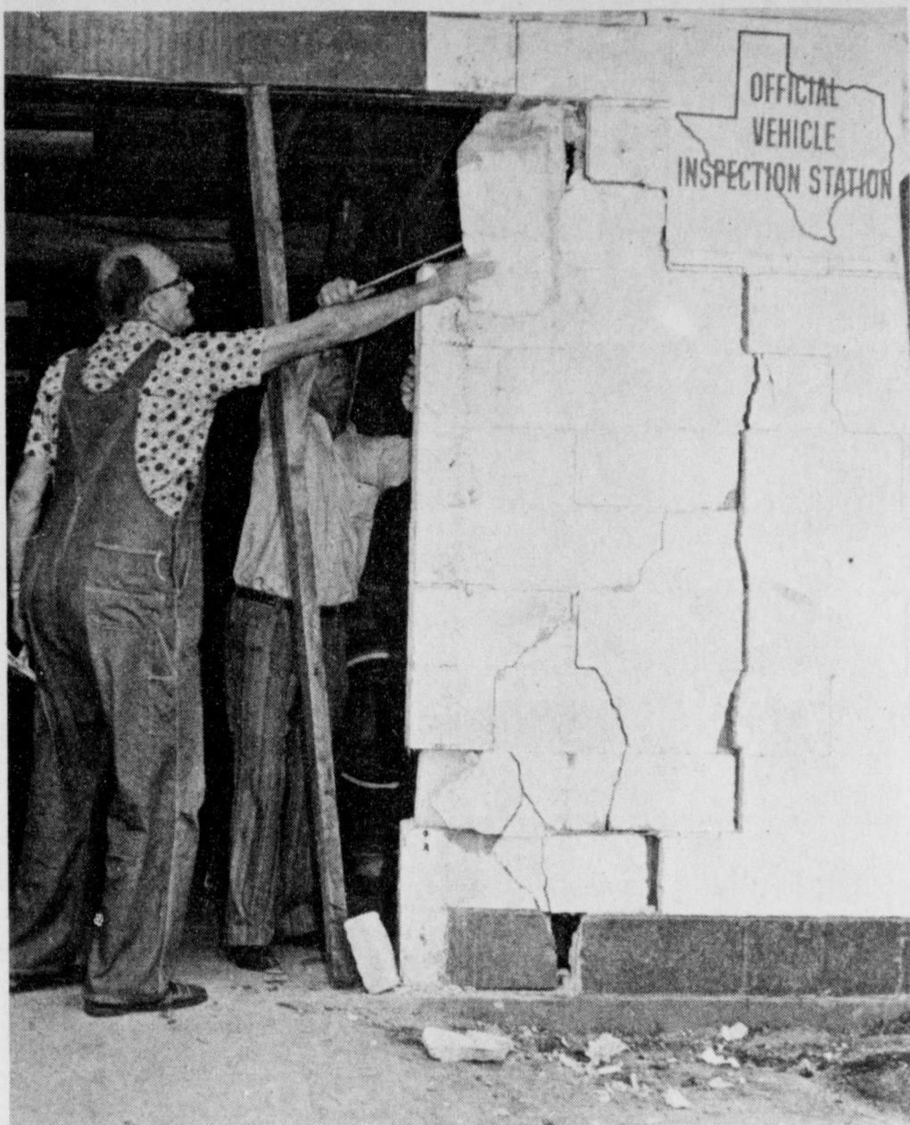
SLIGHT MISCALCULATION —The shop entrance to Roach Butane and Service Station in Deport was damaged when Cleve Stewart of Bogata missed the opening and drove into the wall. (Staff Photo).
