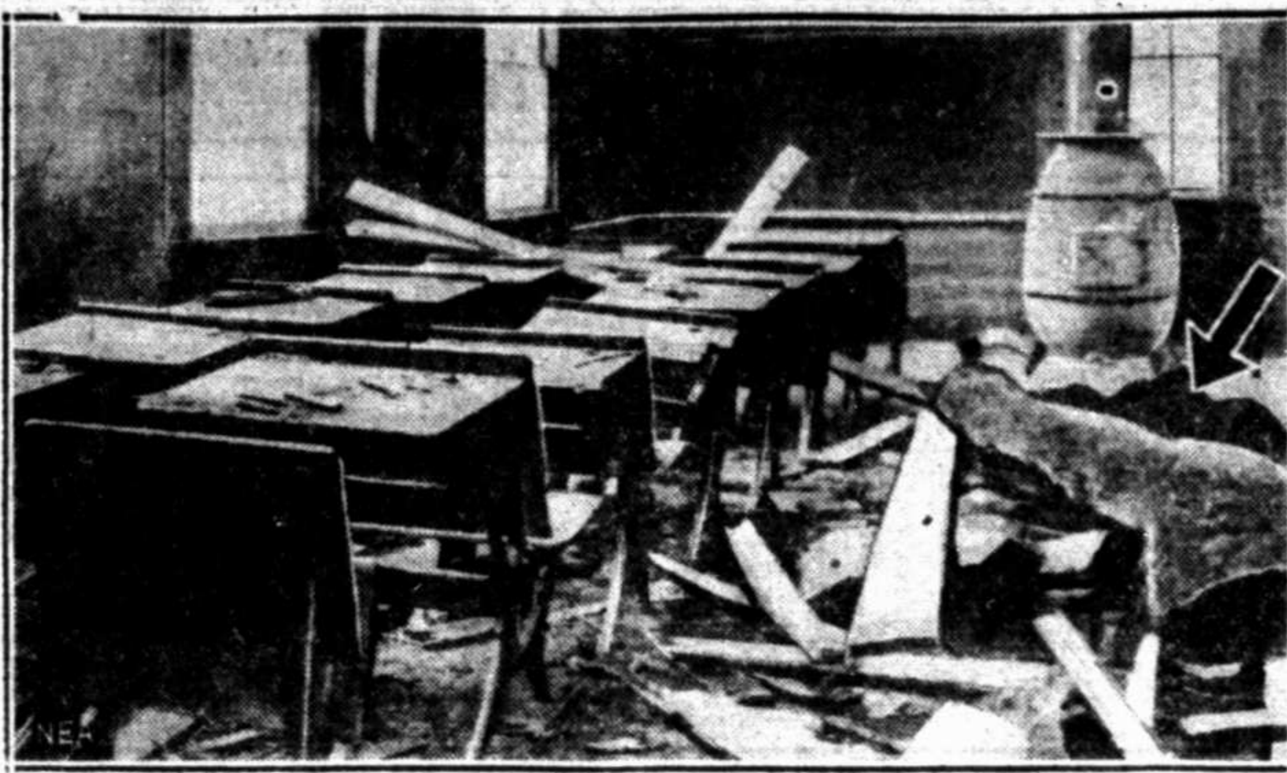
This picture shows how a rural school at Ironton, Ohio, was wrecked when workmen on a nearby highway project set off a charge of dynamite under a tree stump. The explosive hurled the 400-pound stump high into the air and it crashed through the school roof. One boy, James Dean, 12, was killed and six others were hurt. The arrow points to the stump.
