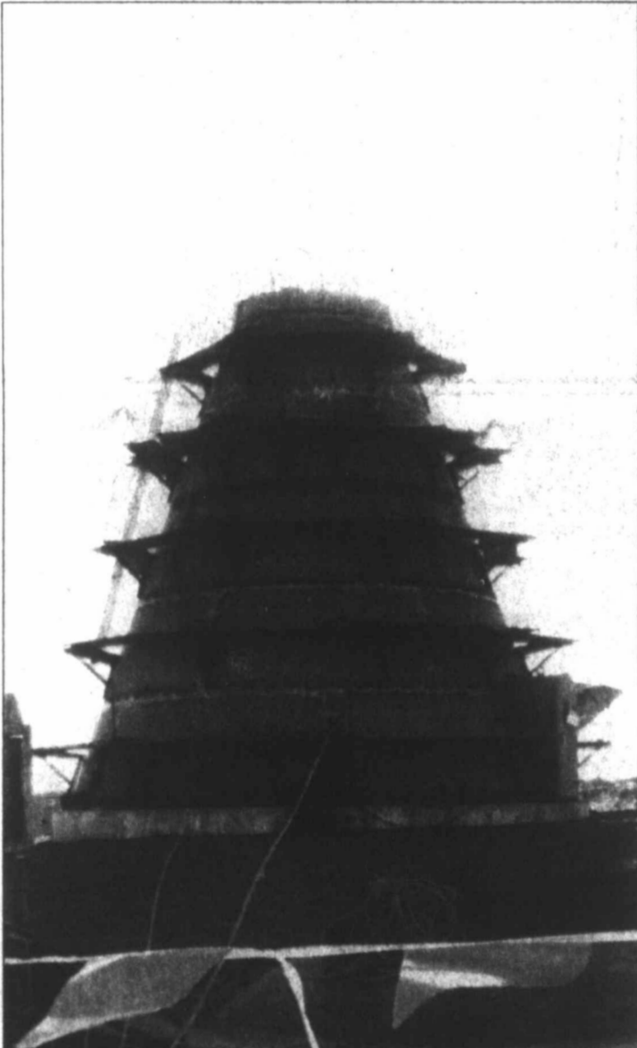
GOING UP - Construction is underway on the north side water tower, located just south of the City Landfill. Once completed, the elevated water storage will hold 350,000 gallons of water. The tower is expected to be raised later this week.
