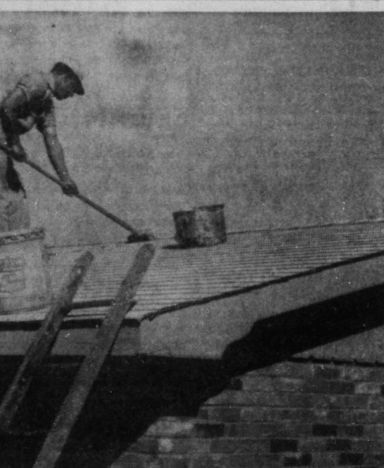
UNIFLEX COATING BY WADLEIGH ROOFING SERVICE —Even the best roofs need care in West Texas weather, Jim Wadleigh, agent for the Uniflex Colored Aluminum Roof Coating in Snyder, tells his customers. Above, Luis Carrisalez gets set to put a protective coating on a roof, a coating that will stay soft underneath a hard top surface, a coating that will add years to the use of the roof.
