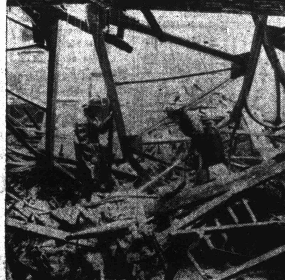
Firemen inspect the ruins of the Lynn, Mass. Classical High School after a 400,000 fire swept through the structure. Six firemen were injured in the five-hour battle to hold the blaze.
