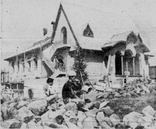
THE EASTERN TOUCH — Workers eat alongside a characteristic Russian building under construction near the Olympic Games sites in Rome. It will house a Russian-style restaurant catering to visitors to the giant sports festival this summer.
