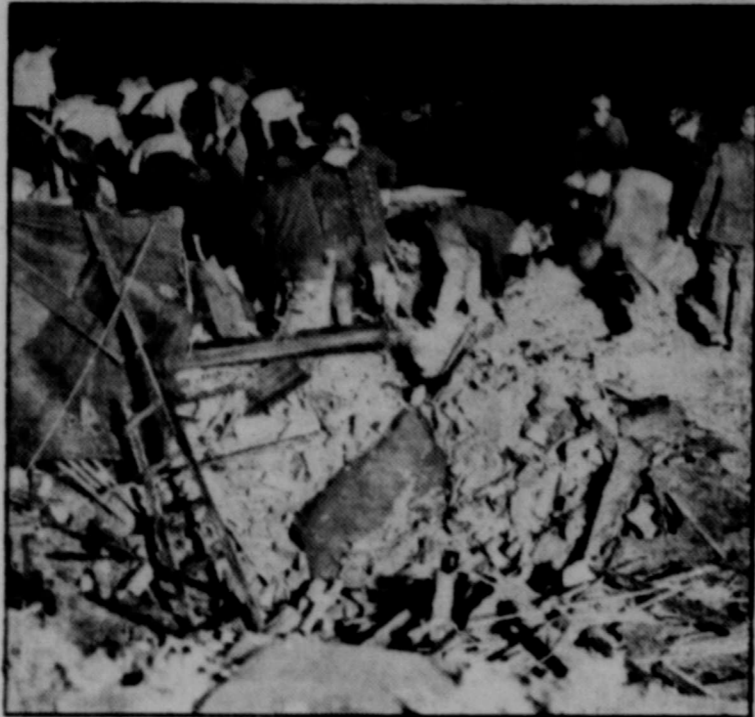
New York firemen and police are shown above as they searched for victims in the ruins of three Staten Island tenement houses which collapsed during a violent rainstorm. Caught without a chance to escape, 19 people were killed and many others injured when they were buried under tons of bricks and debris.
