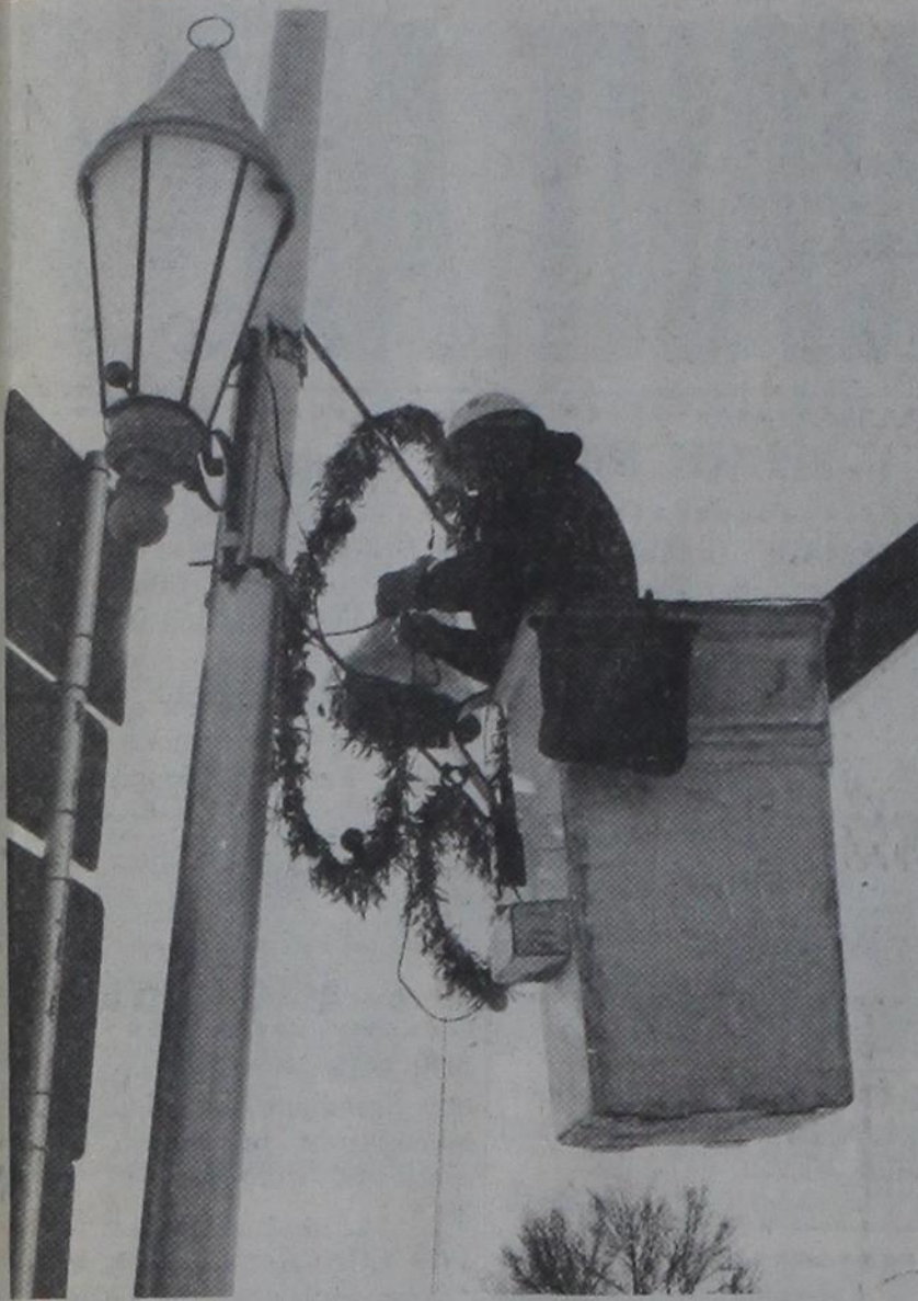
LET THERE BE LIGHTS—Bob Murdock of Southwestern Public Service Co. works from a sky-bucket to hook up one of Dimmitt's downtown pole decorations. The Yule decorations were assembled and installed by members of the Dimmitt Volunteer Fire Dept.
