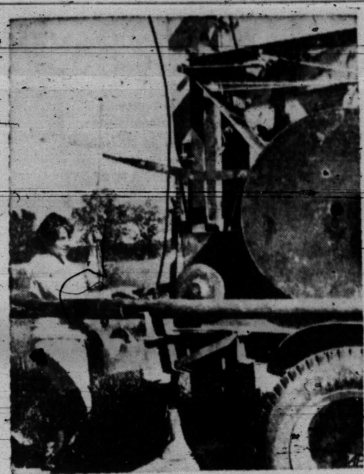
CAPABLE CONNIE AT THE HELM —Connie Catlin, 19, of Eyoia, Minn., is a capable young lady when it comes to handling a well-drilling rig. Working for her father, Casey Catlin, she has run well-drilling rigs during the summers since she was a high school freshman. She expects to start college at the University of Minnesota in Duluth next fall. She got into the unusual occupation, Connie says, "because there wasn't a boy born first in our family." She can handle the whole job, from starting to the final gush of water. (AP Wirephoto)
