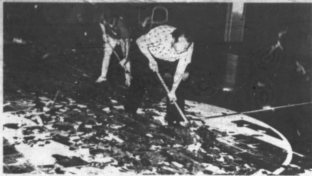
WALLACE CENTER PROJECT of Colorado City's Jaycees is pictured here as two Jaycees, Frank Kantro and Don Banta, work taking up the tile floor at Wallace gym in order to use the area for a skating rink. When the tile is removed, the concrete floor will be finished and smoothed for roller skating.
