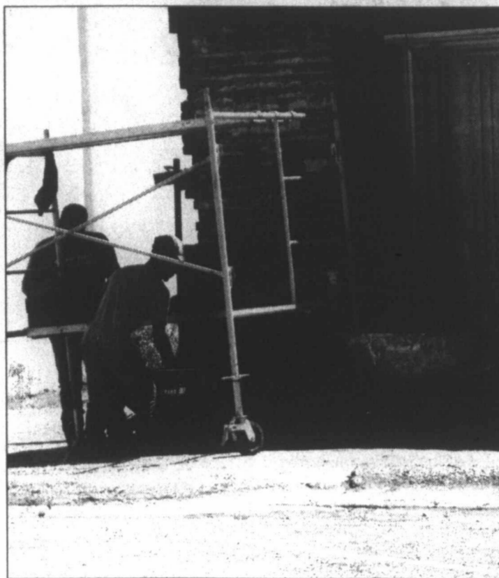
USING THE NEW TO PRESERVE THE OLD – Masonry crews were hard at work Monday on the building that houses Bigg's Pizza. The crews were putting up bricks on the outside of the building located on 2 nd Street downtown. The work is part of restoration of the façade of the building to make it look like it did decades ago.
