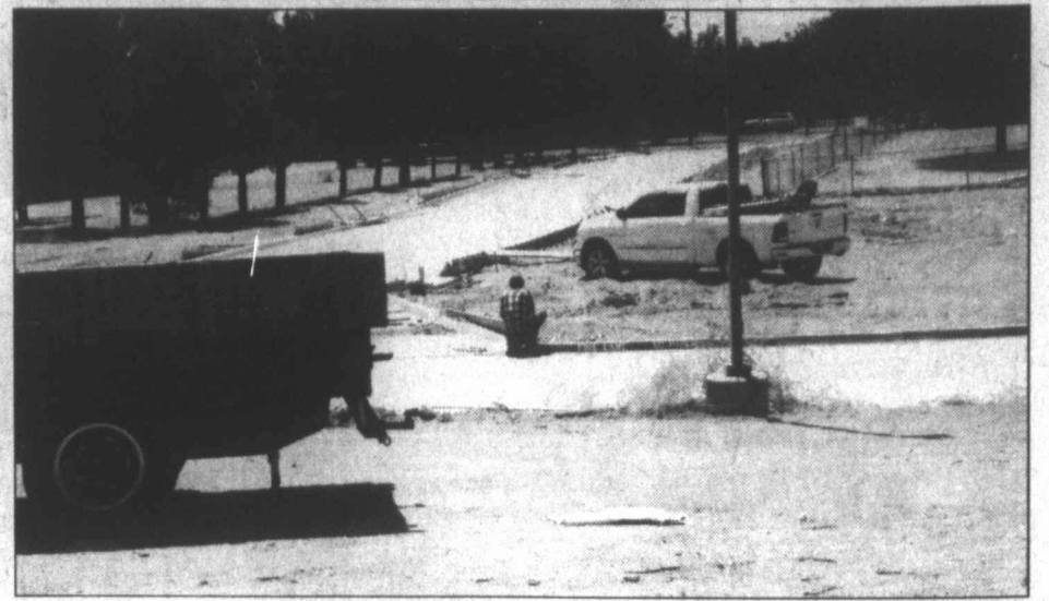
BUS ROUTE - Crews could be found working on curbing on the newly paved extension of 13th Street. The street was extended from Eastover to the west side of the new CISD campus to allow for an alternate route for bus traffic.
