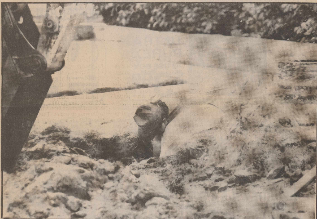
IN A MUD HOLE: Randy Martin, Rotan City employee, was up to his elbows in water last Tuesday morning attempting to fix a broken 2 inc water line just North of the First United Methodist Church.
