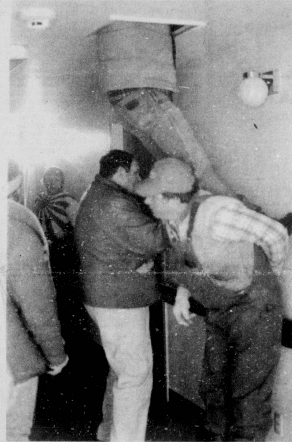
THE CENTRAL HEAT unit had some burned wires in it at Red River Haven. All three fire trucks responded. Many volunteers in Bogata rushed to help evacuate patients if necessary. The staff had already removed patients from the wing where the smoke was found. No fire was discovered. (Staff Photo by Diana Eudy)
