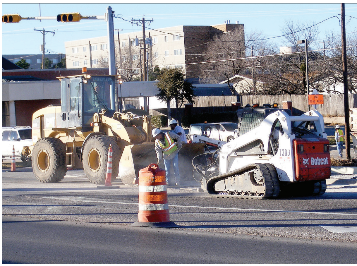
Work crews tear up the old surface on Gregg Street at the 15th Street intersection this morning. Renovation of Gregg is expected to continue for the next few months.
