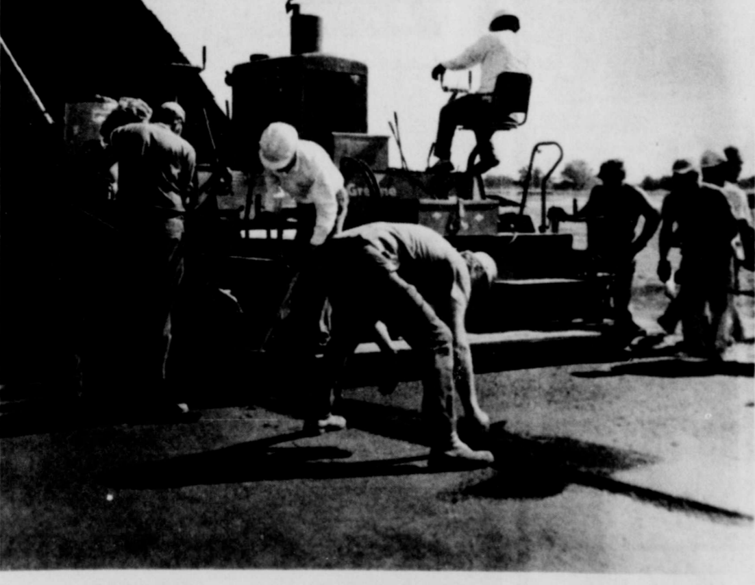
LAYING NEW TRACK--Workmen are shown as they lay the new reslilt track at the high school, Friday. The men completed the stripping and finished touches to the track Tuesday. After a "curing" time of some 60 days the track will be ready for service.
