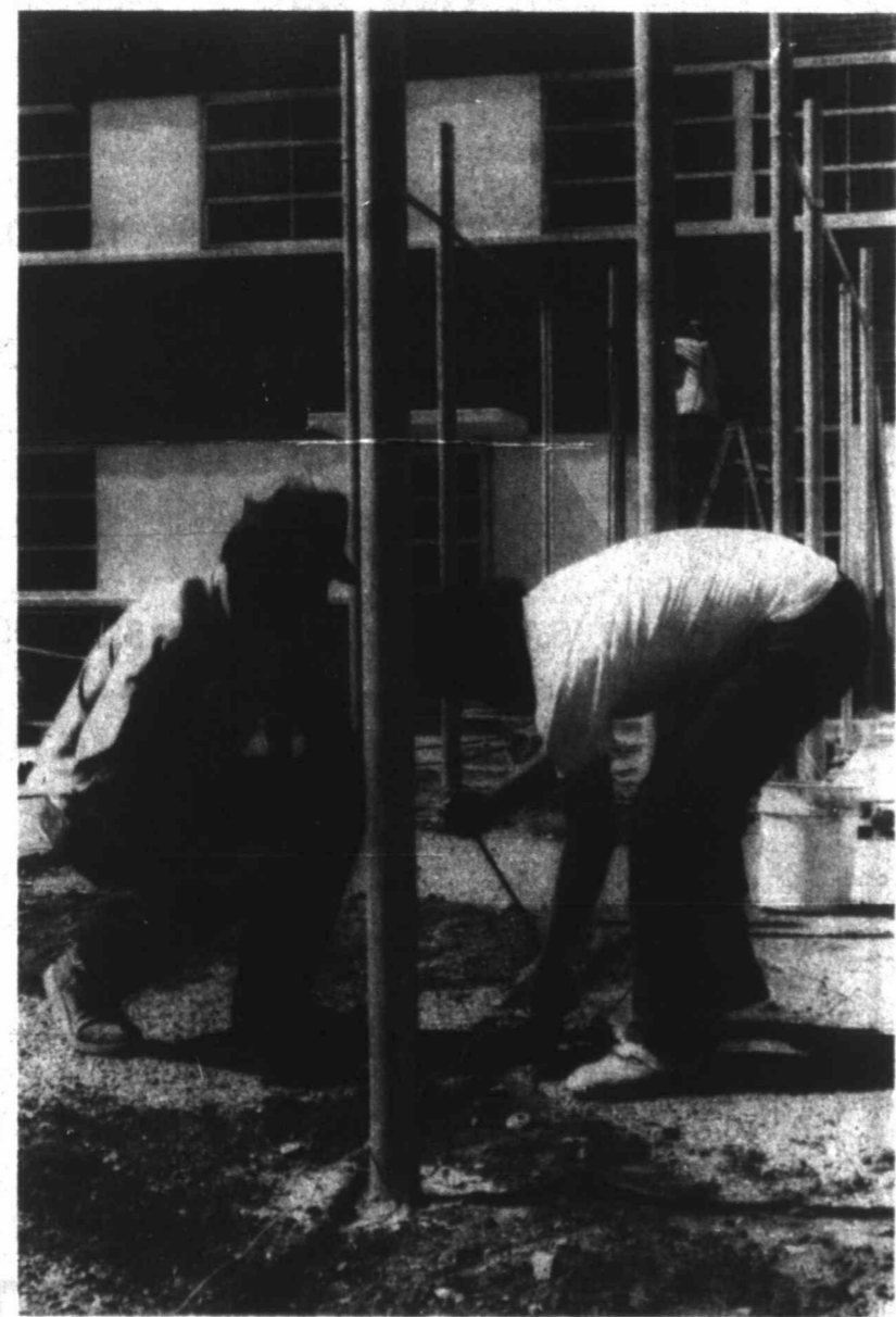
FENCING IN THE EXERCISE AREA: Workers from the American Fence Co. out of Odessa have been working this week fencing in the exercise area just east of the Mitchell County Jail. This work started Tuesday and is expected to be completed in about a week. The exercise area was needed to comply with the Texas Jail Standards.
