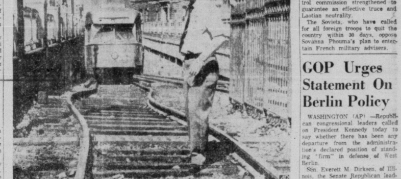
TWISTED RAILS—When the heat hit 95—the highest mark of the year in Boston—this is what happened to MTA tracks. Despite the heat-warped rails cars were able to move slowly over the roller-coaster section. (AP Wirephoto)
