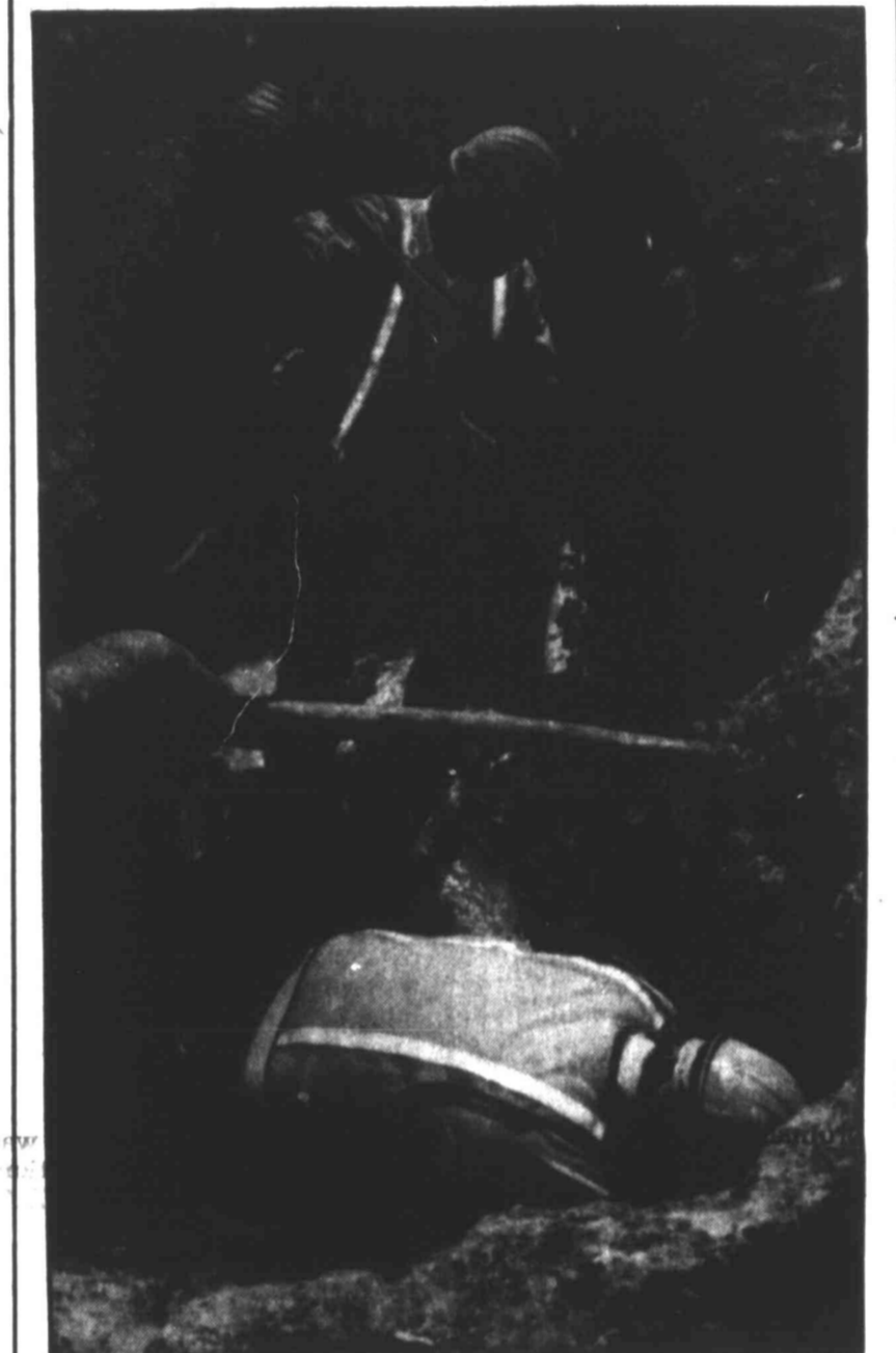
City of Big Spring workers dig in a trench as they were putting in a new water valve along West 16th St. Tuesday. Several valves were installed at different locations along the road.
