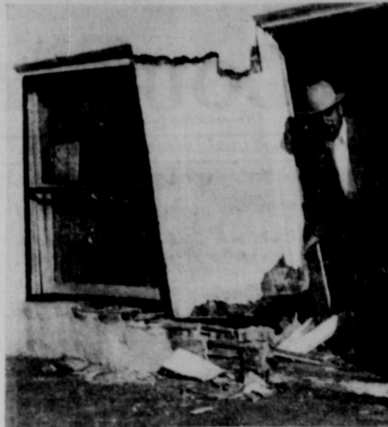
A SLIGHT MISHAP—John Mayfield, Chamber of Commerce manager points out a slight flaw in the wall of the Chamber building on South Main after Mayfield let a pickup run into the front of the building on his way to get the Cash Day tickets from the building. The building has been repaired and now everybody's happy.
