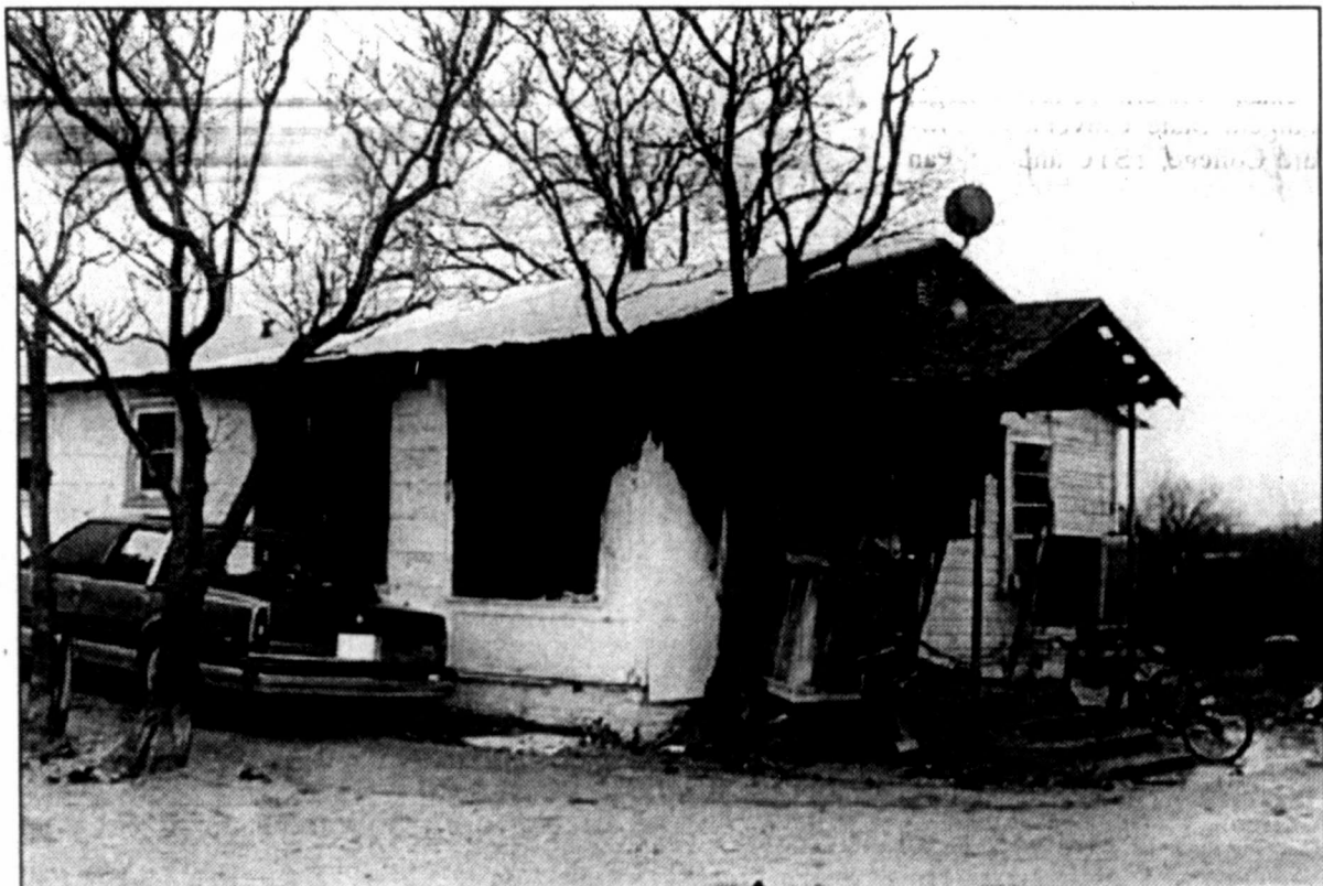
A MIDNIGHT MONDAY FIRE made a total loss of the 265 Wallace St. home of Frances Emerson in southeast C-City. Ms. Emerson and a grandchild escaped unharmed when an apparent electrical short in the living room ignited the blaze. Ten volunteer firemen in three trucks responded at 11:56 p.m. and were at the scene until 2:16 a.m. Tuesday.
