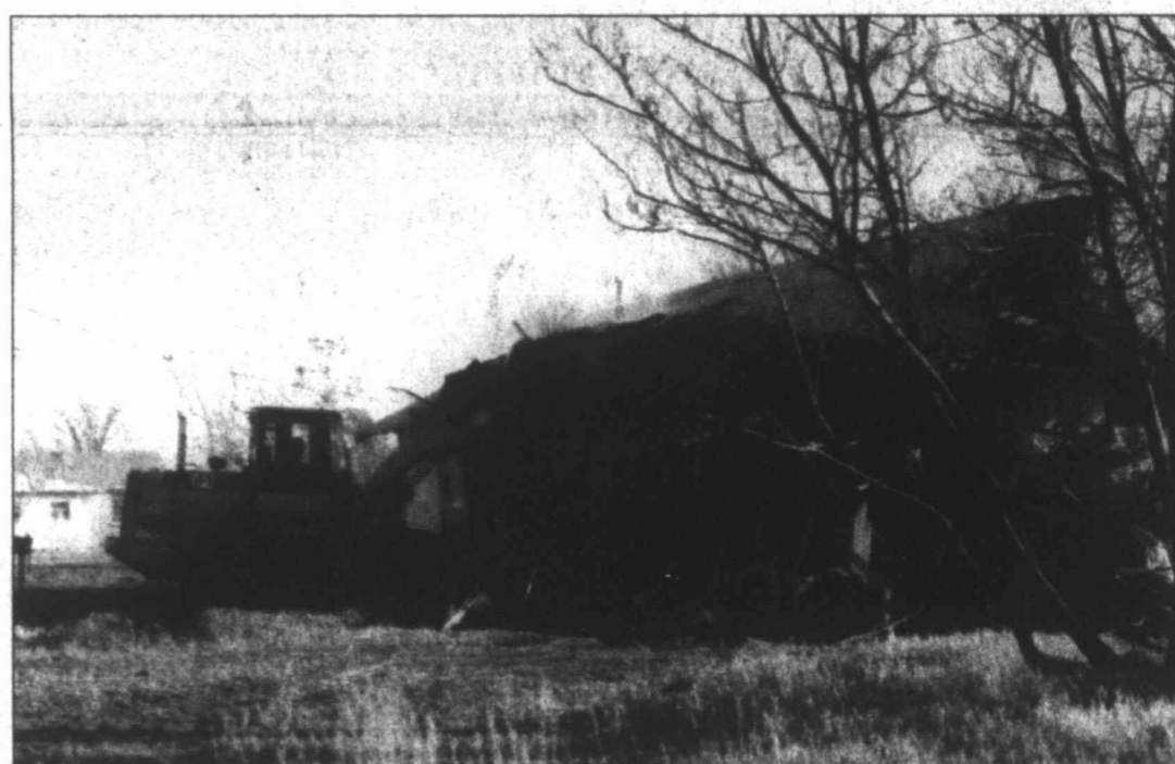
UNSAFE STRUCTURE - The former home of Hailey Dunn on Chestnut Street was demolished on Monday last week. The structure was inspected and deemed unsafe by the city and was torn down to prevent anyone being hurt by entering the house.
