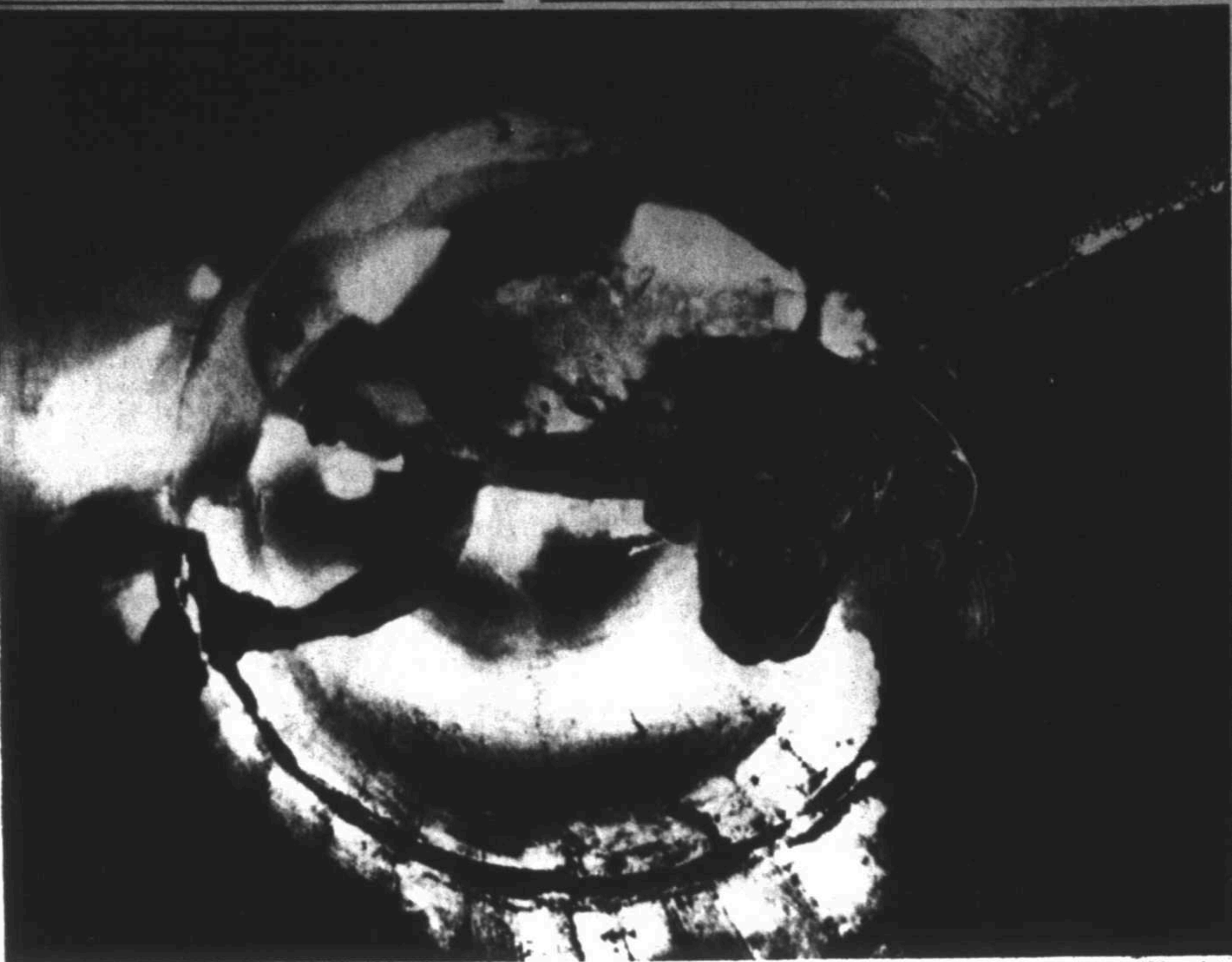
Marty Chamberlain uses fast-drying cement to patch a water line that runs for a half mile, 20 feet underground, between a filtration plant and a pumping station in Grand Rapids, Mich. "It's really interesting work, as long as you're not cursed by claustrophobia," said the Grand Haven man, who refers to himself as a "water rat."
