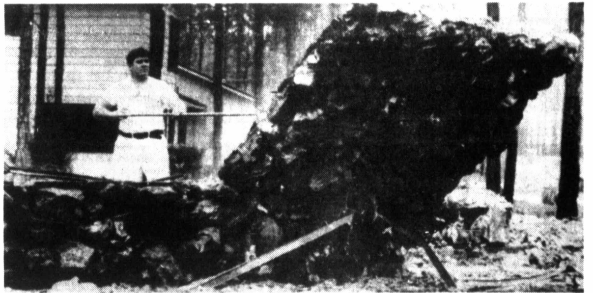
WALLS TUMBLE DOWN — Charles Hanger pushes down a stone wall that used to decorate the front of his house in Palm Coast, Fla., after his home was hit by wildfires over the weekend.
