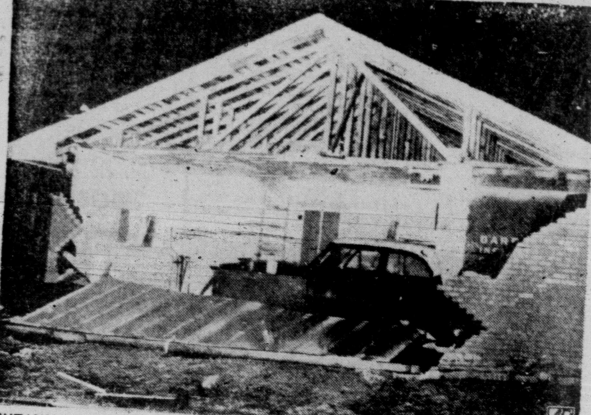
CUTAWAY VIEW—Tornado funnels which passed low over Oklahoma City caused a lot of damage to homes and buildings. Typical is this side view of a home with the roof touched — a 50 mile long strip of central Oklahoma caused widespread damage and 31 injuries. One man in Oklahoma City died, several hours after suffering a heart attack when the 85 miles an hour winds pelted the city, and damaged his home. (AP Wirephoto)
