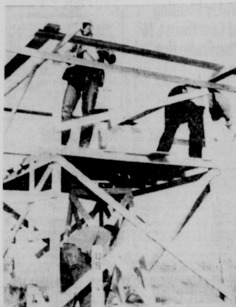
BUILDING THE TOWER—Three members of the geodetic survey party in Perryton are shown building a 10-ft. wooden tower for use of the light and instrument survey party. Ed Skupa, Charlie Call and Stanley Husted put up one of these towers a day.
