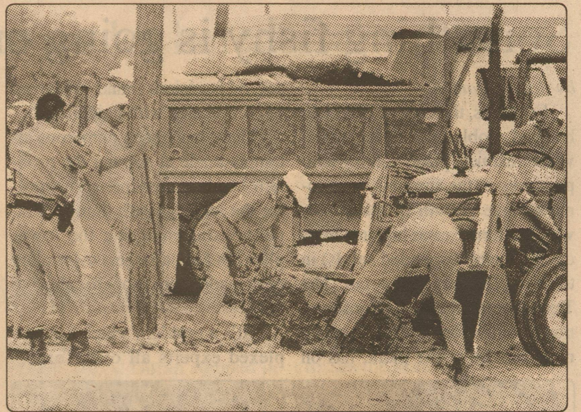
Hard labor — Field Corrections Officer David Olivan supervised an inmate work detail recently as they removed a portion of the old sidewalk beside the Schleicher County Library.
