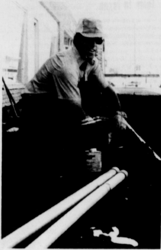
CARLIS BILLS--former Earth resident is doing the electrical work on the new bank building.
