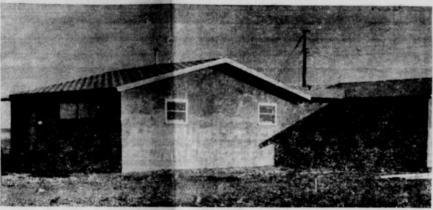
SEVERAL NEW HOMES ARE UNDER CONSTRUCTION — In Earth making the prospects for the approaching New Year look progressive. Pictured almost completed is the Bobby D. Green home in North Earth, built by Bob Ussery.
