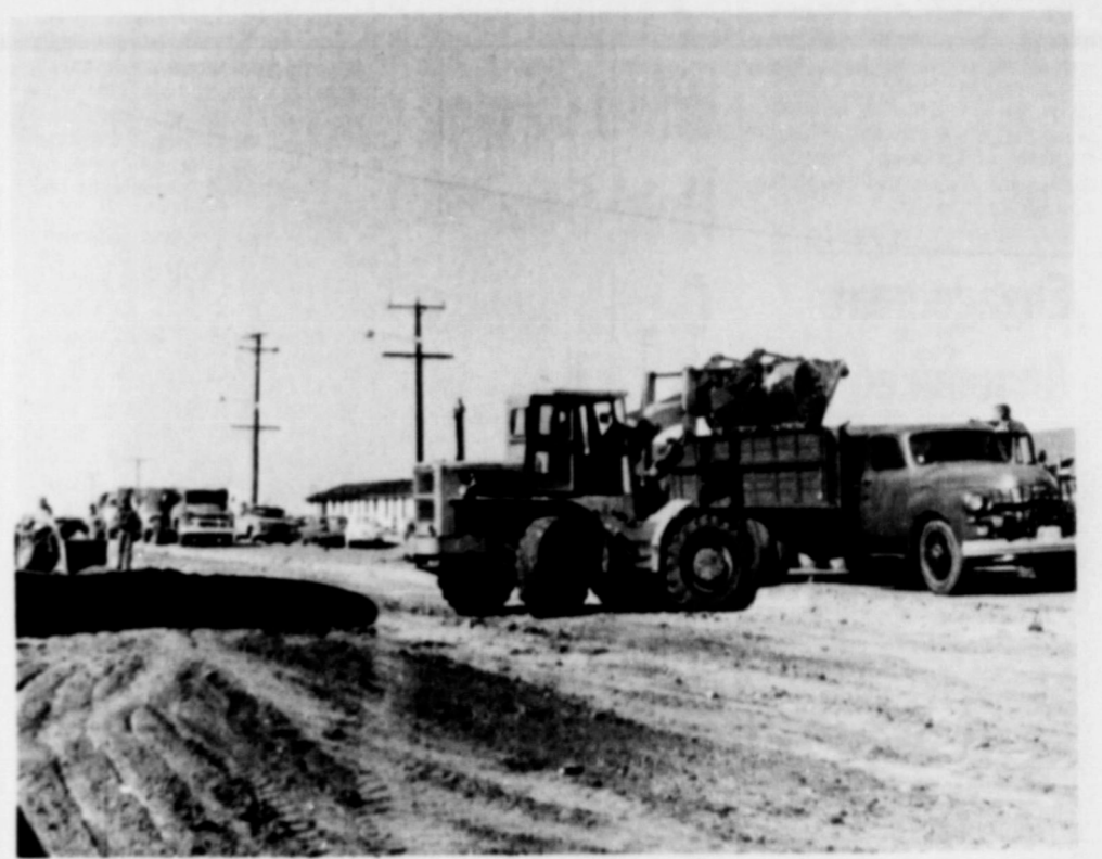
SEVERAL MEN in the Springlake school district undertook a caliche hauling project last week preparing parking space, north of the new school lunchroom for paving, which will be done, when the weather gets warm enough.
