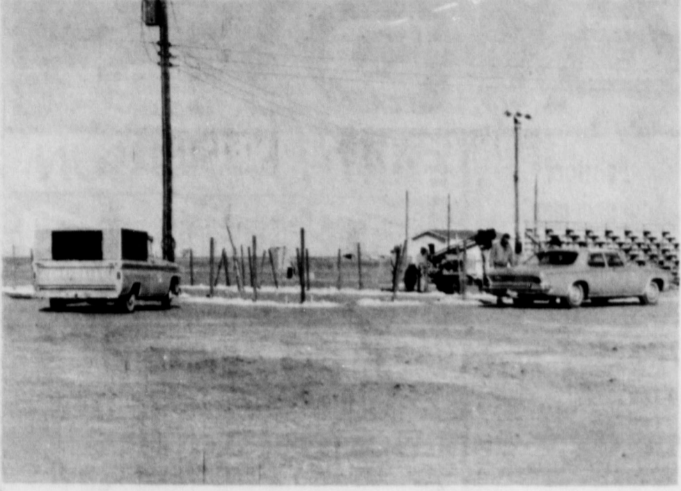
WORK IS UNDERWAY on rebuilding the Rodeo ground arena. The old arena and shoots have been torn down and will be replaced with a concrete tile two story structure, housing a concession stand and judges stand. New posts and fence are also being put up.
