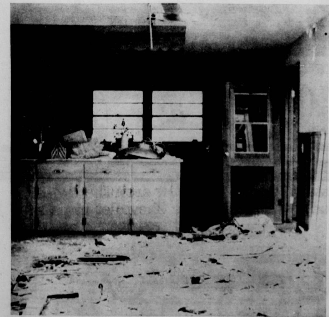
THE HOWARD BRIDGES LOVELY HOME — Where twelve ladies were gathered for singing while their husbands attended the church meeting. Pictured is the den and kitchen of the house which is unroofed. The ladies, all grouped in the living room. Damages were much lighter in the
