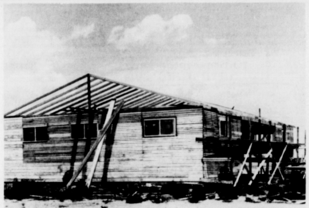
THE SCOUT HUT is under construction in the City Park and promises to be a nice meeting place for Scouts when completed.
