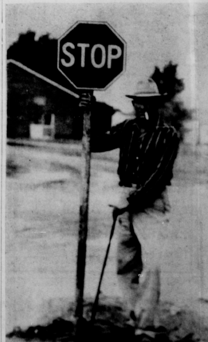
STOP SIGNS — Are being erected on main traveled streets. Putting up the sign is W. F. "Dunk" Williamson, City Water Superintendent.
