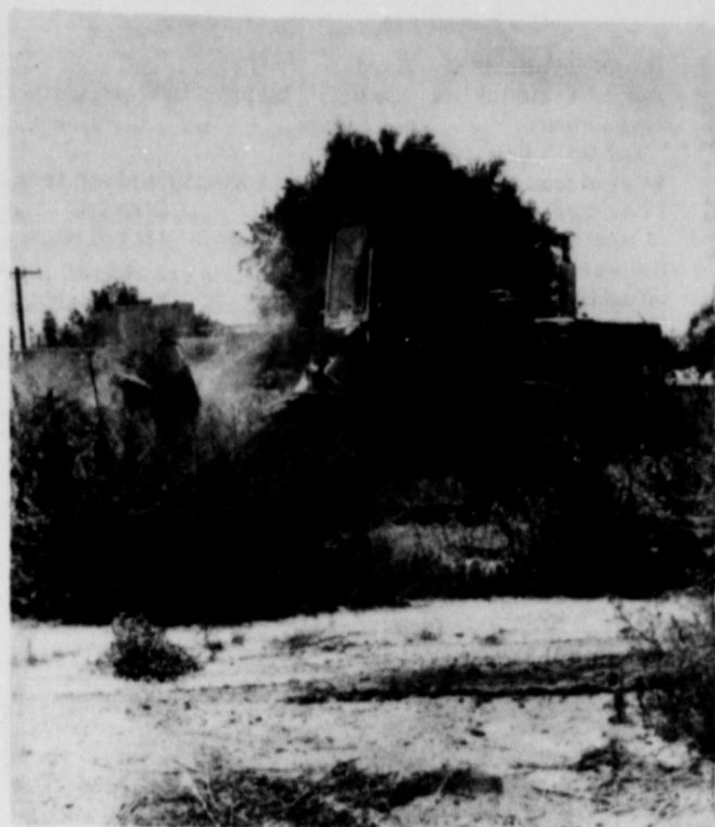
MAINTAINER CLEANS ALLEY... Monday afternoon the county maintainer was put to good use cleaning the alley of piles of debris collected as construction of the lovely bank building moved along. Some of the weeds are also missing along the alley.
