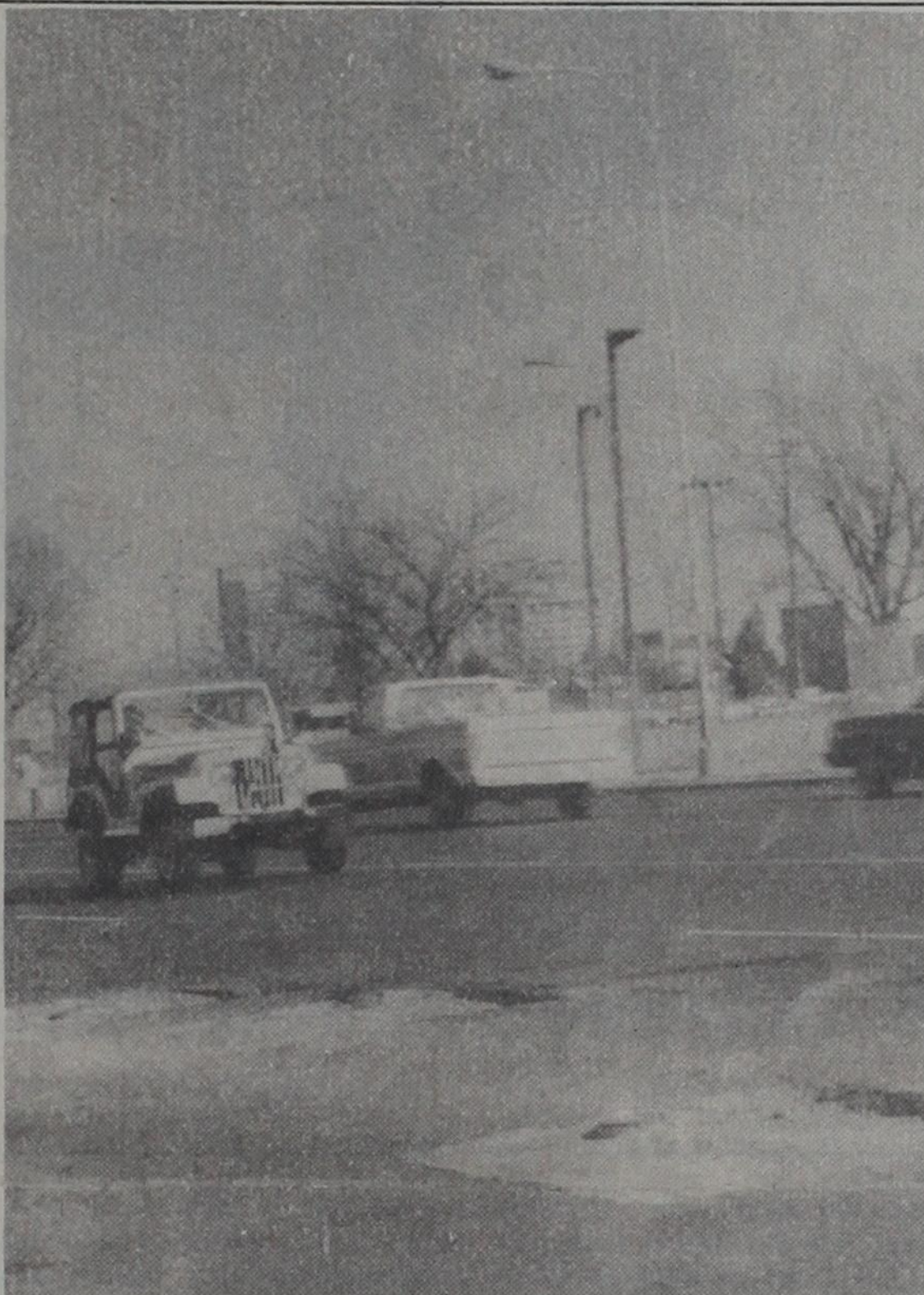
BUMPS AND GRINDS —Motorists on Avenue Q had to dodge patches of road surfacing removed by city crews to raise valves for sewer and water lines. The bumpy ride was the result of a highway department experiment to determine the best way for leveling the street around the valve hatches. City crews were expected to fill in the patches of removed surface by Thursday. (Times Photo)
