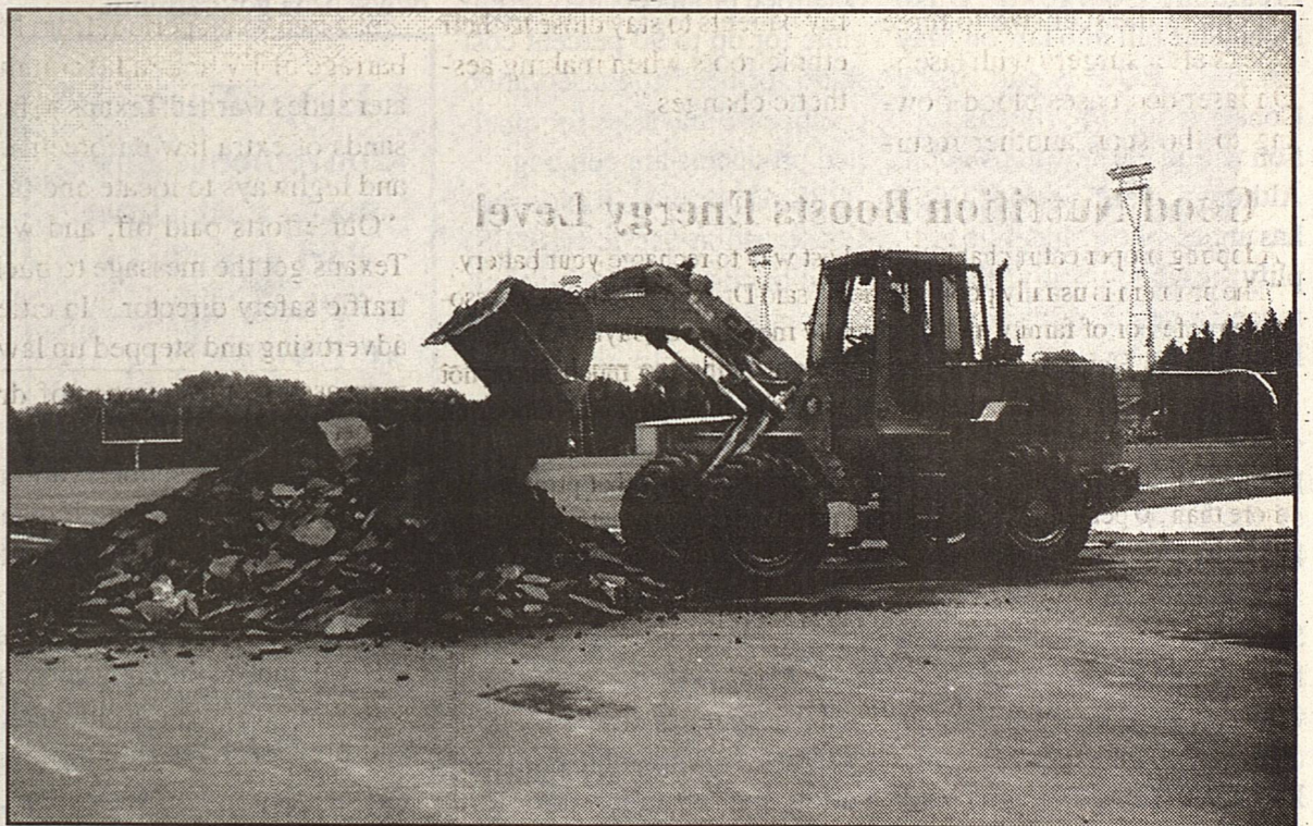
Precinct 4 employee Junior Rivas mans a front end loader scraping up old asphalt on the Plains ISD running track. After 20 years of excellent service, the old track deteriorated to the point it had to be replaced. Contractors are scheduled to start laying the new surface within a few days.
