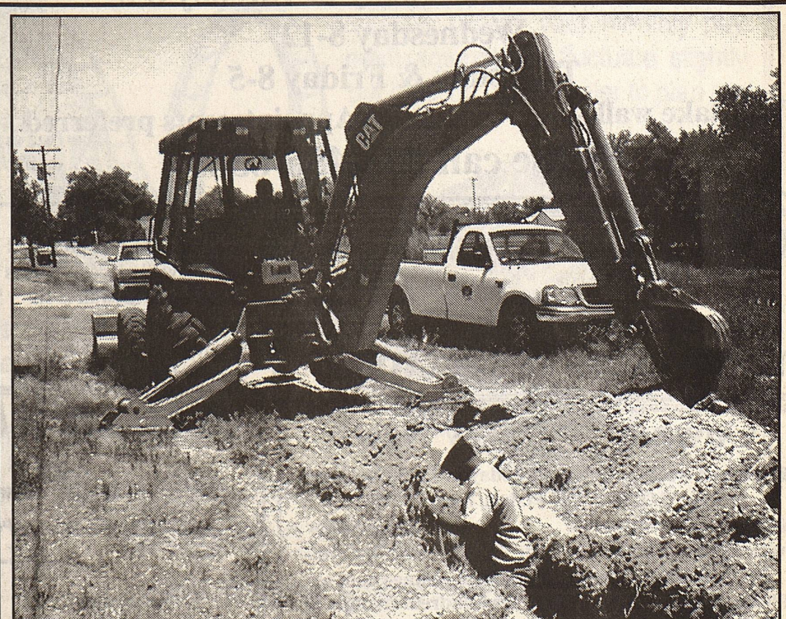
City employee Alex Bariantes, in backhoe, and summer student employee Ryan Martinez were busy last week preparing to lay a new water line in the alley between 3rd and 4th streets. The old two inch line will be replaced with a four inch line, providing residents with more water volume and pressure.
