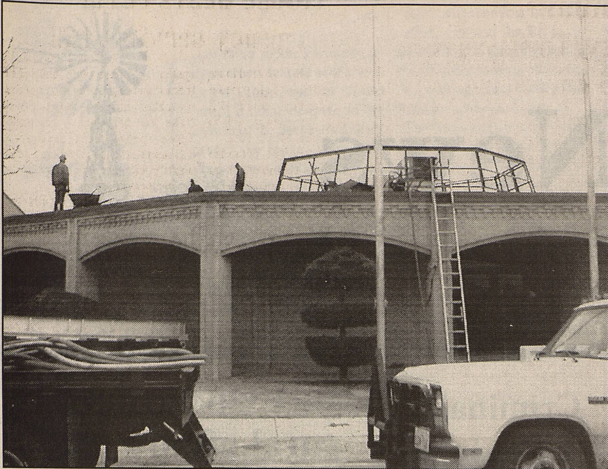
These workers braved a cold and very blustery morning last Saturday, re-roofing and repairing the roof of the Plains ISD Learning Center building.
