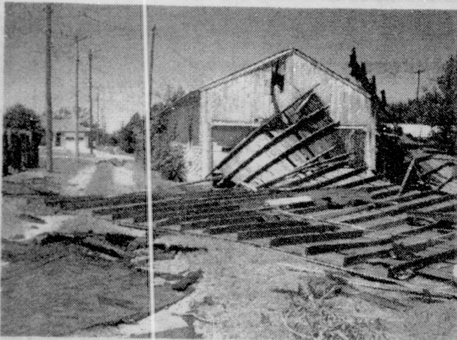
The roof from Windom's Auto Supply sadly lays upside down in a nearby yard. Notice the hole near the peak of the garage where a 2x6 was driven through the sheeting.
