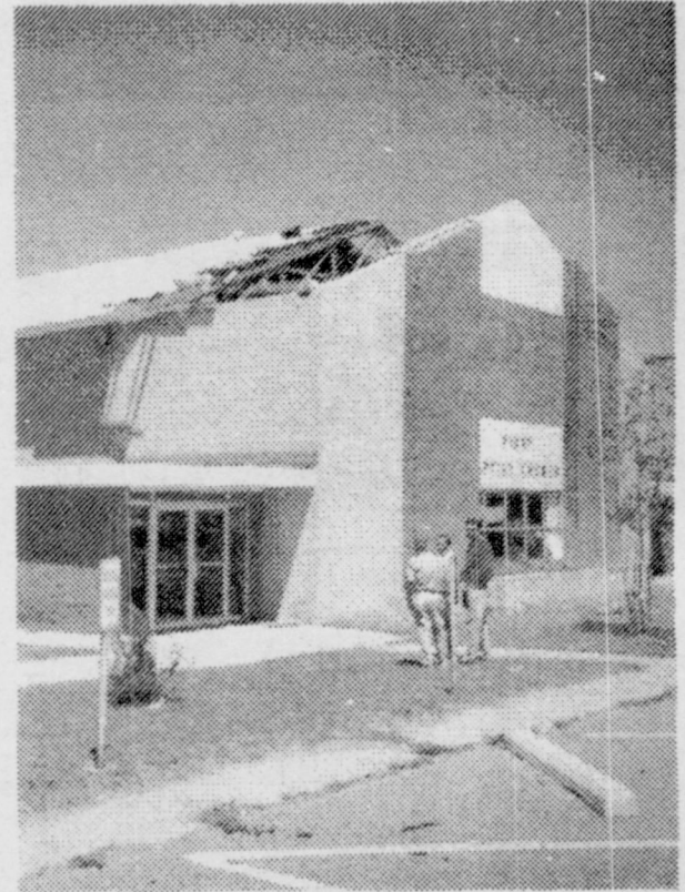
The First Baptist Church suffered roof damage. Repairs are being made as quick as possible to get the building back in shape, hopefully in time for graduation.
