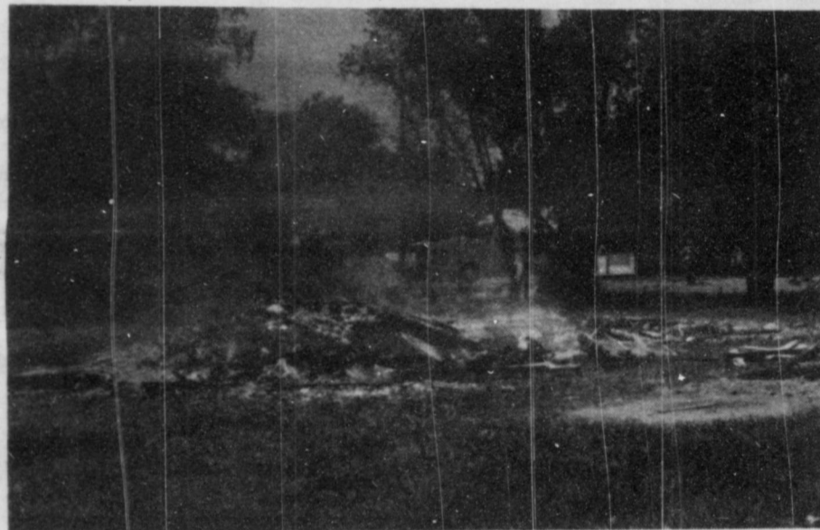
Fire takes care of this demolished house in a staged controlled Fire Drill by Volunteers.
