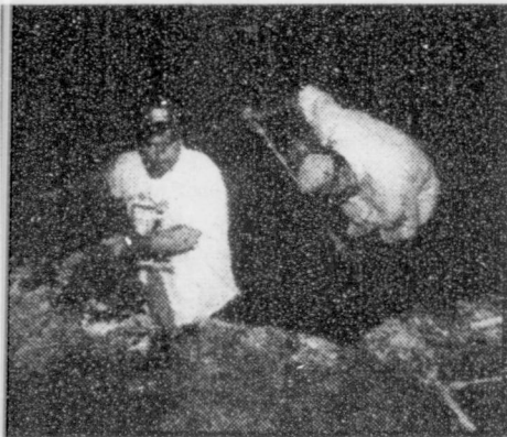
City employees Bill Anderson and Chet Bohlar excavate the damaged water works to repair the leak.
