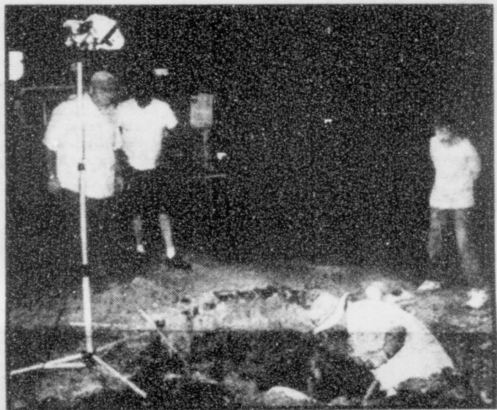
City employees work past midnight to repair a major water leak on Commerce Street.
